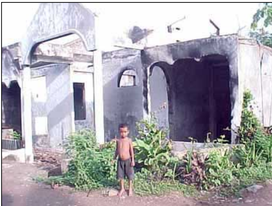
The charred remains of buildings are still a common sight throughout East Timor sixteen months after the referendum.
