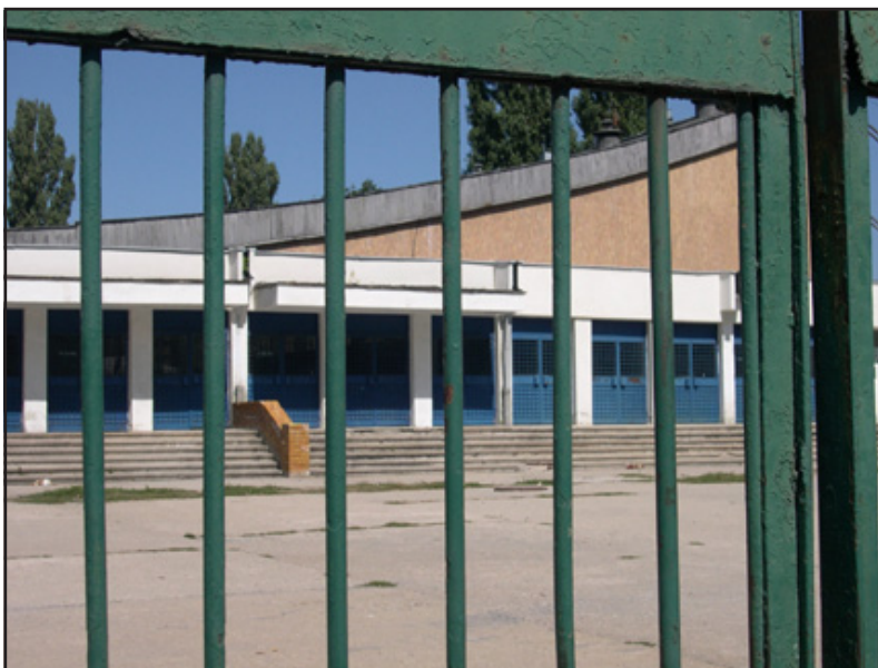
The Romanian hockey team has not been able to use the Lia Manoliu ice rink, whose roof still leaks.
