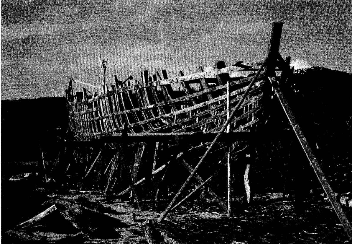
Above: Framework of the hull of an Anguillan boat, forty feet in length made by hand by some of the most famous boat builders in the Caribbean
