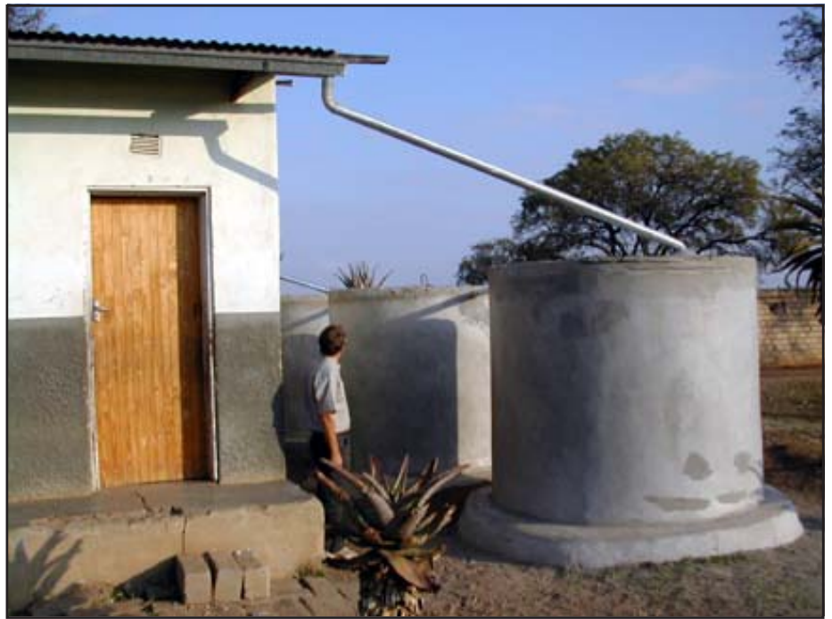
‘SSP’s School Project.’ (...gutters to 10,000-liter rainwater harvesting tank.)
