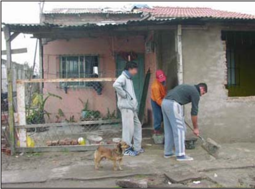
These men receive Planes Trabajar through the CTA-Solano and are contributing their labor for repairs and improvements to this home.
