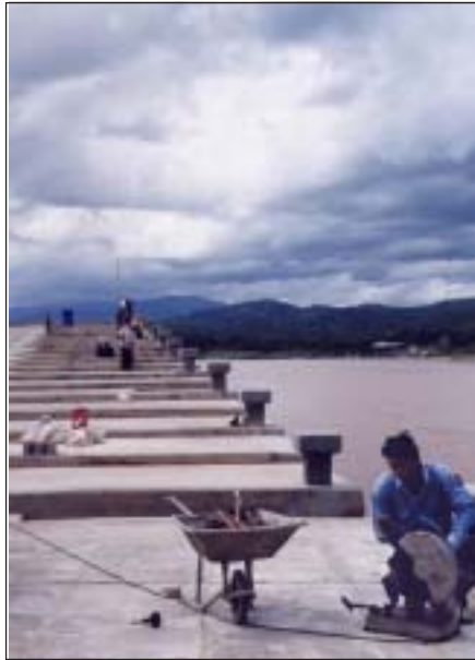
Finishing touches made to Chiang Khong's new port in Hua Wiang. This port threatened to put the Wat Luang laborers and boat operators out of business.
